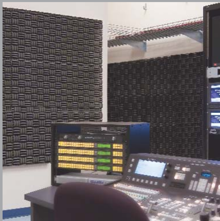
SONEXclassic™ Panels in charcoal colortec used in control room of broadcast facility.
